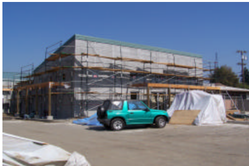
Friends of Children with Special Needs "Dream Center" under construction in September 2005.
